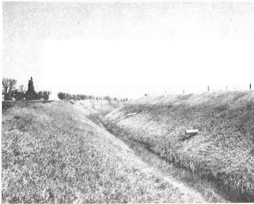
Figure G-1. Example of a well maintained open drainage channel.
