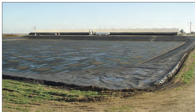
Figure 3. Geo-synthetic cover installed on a manure storage. Edge of the geo-membrane is typically trenched in. Note, these covers are not to be walked on and the storage should be surrounded by a fence.
